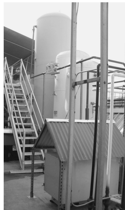
Kunde Winery installed a new 15hp air compressor to replace a 50hp compressor and added a second, larger 2,560-gallon air holding tank to the existing 1,670-gallon tank in 2004. The increased air-holding capacity allows a smaller air compressor to run less often while maintaining a constant pressure.
